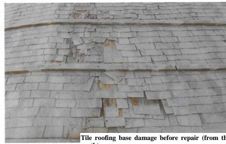
Tile roofing base damage before repair (from the north)
